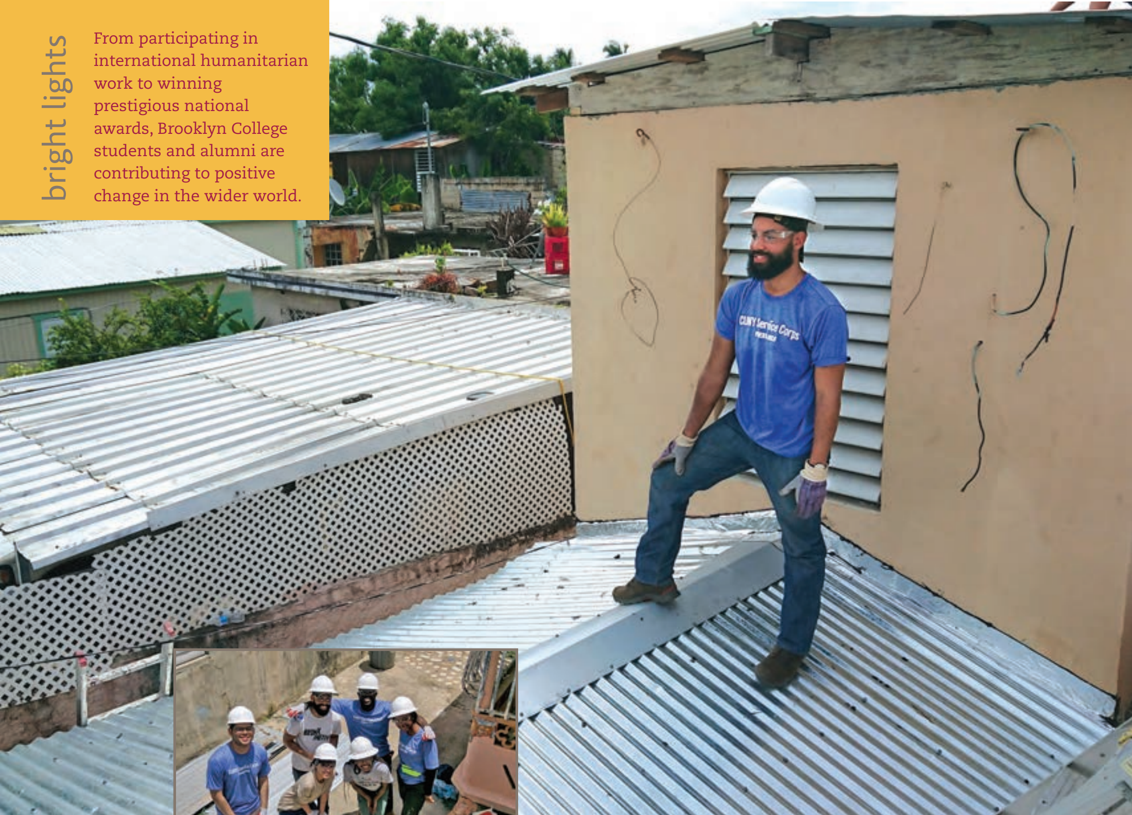
Jonathan Cabral works atop a roof in Puerto Rico, where he helped rebuild homes in the aftermath of Hurricane Maria with CUNY Service Corps. Inset, Cabral with fellow CUNY students.
